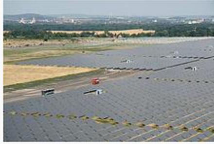
40 MW PV Array installed in Waldpolenz, Germany
